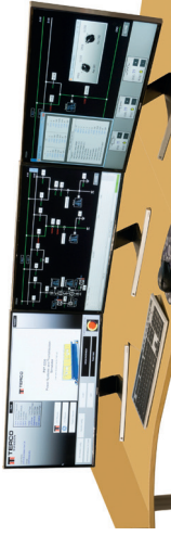
PST2250-15 SCADA System
